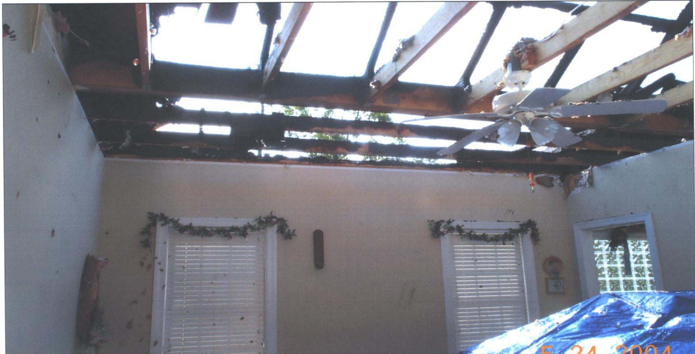
May 23, 2004, Lightning damage to home at 10 Hialeah Place, Pinehurst, NC
