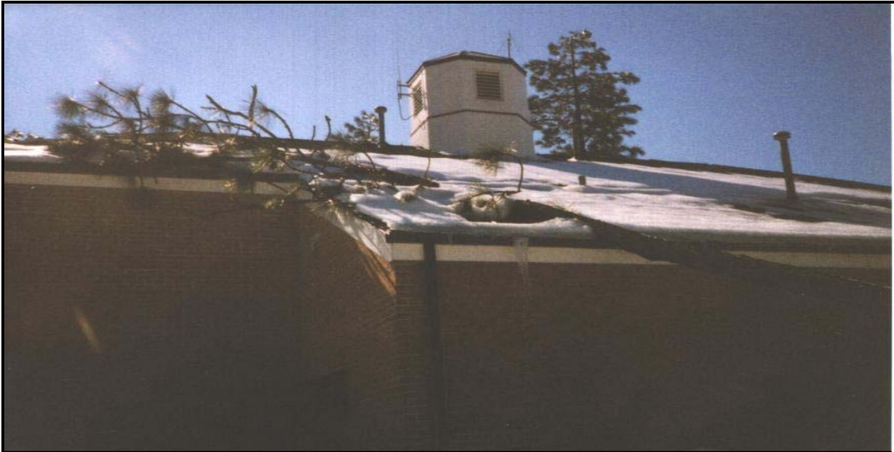
Damage sustained to the Pinehurst Fire Department/2000 Winter Storm.
