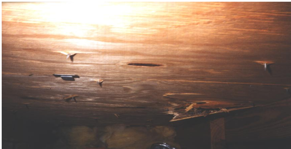
Damage sustained at the Pinehurst Fire Department/2000 Winter Storm
