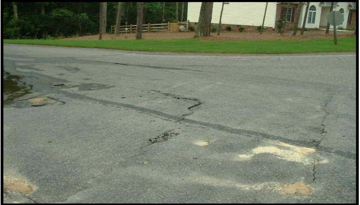
Results of nuisance flooding, Golf Course #6, Pinehurst, NC
